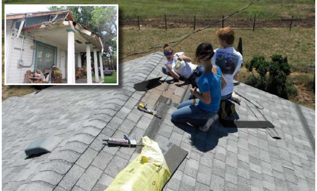
Wesley United Methodist youth help repair wind damage to roof of one house.
